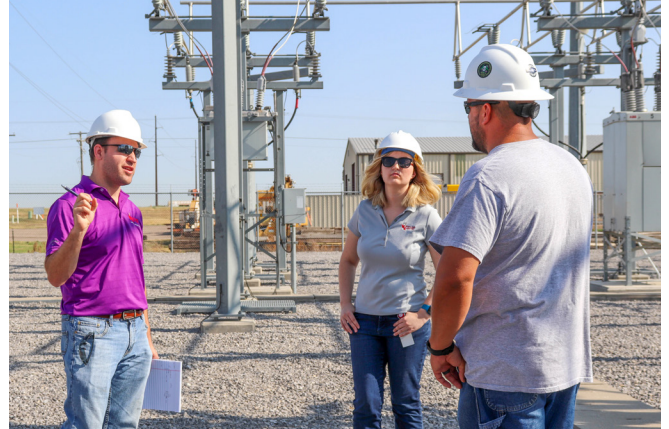
Brandon Barrett, manager of engineering (left), discusses details of the Irsik and Doll substation with Kyle Strickert, substation maintenance foreman (far right) and Nicole Tarpein, engineering intern (center).
