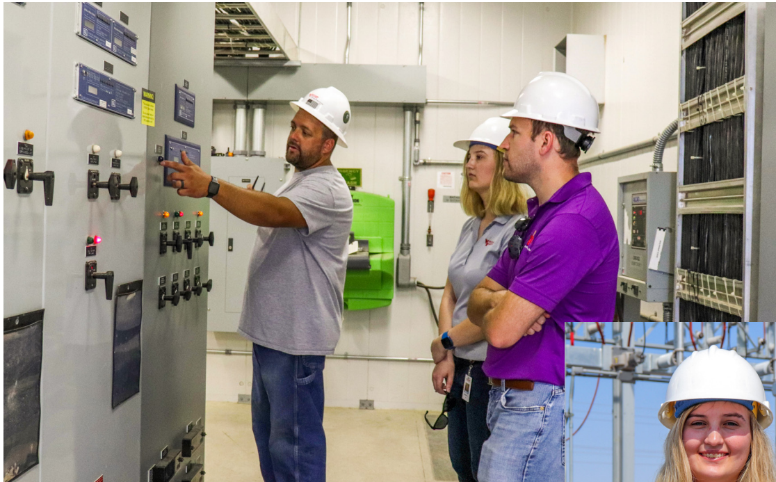
Above: Kyle Strickert, substation maintenance foreman (left), explains control room operations inside at the Irsik and Doll substation in Finney County. Also pictured are Nicole Tarpein, engineering intern (center), and Brandon Barrett, manager of engineering (right).
